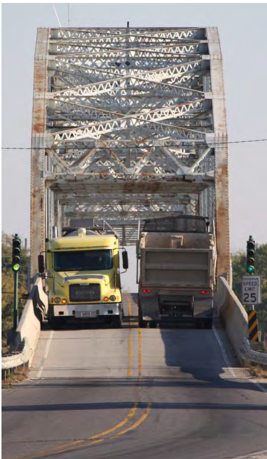
The narrow travel lanes and lack of shoulders on the Chef Menteur Bridge.
